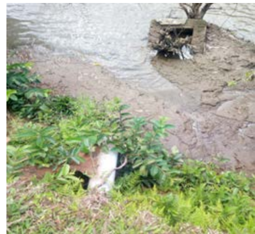
Plate 5: Broken Down Waste Pipe
