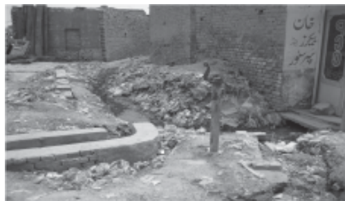
Figure 4: Blockage of open drains
